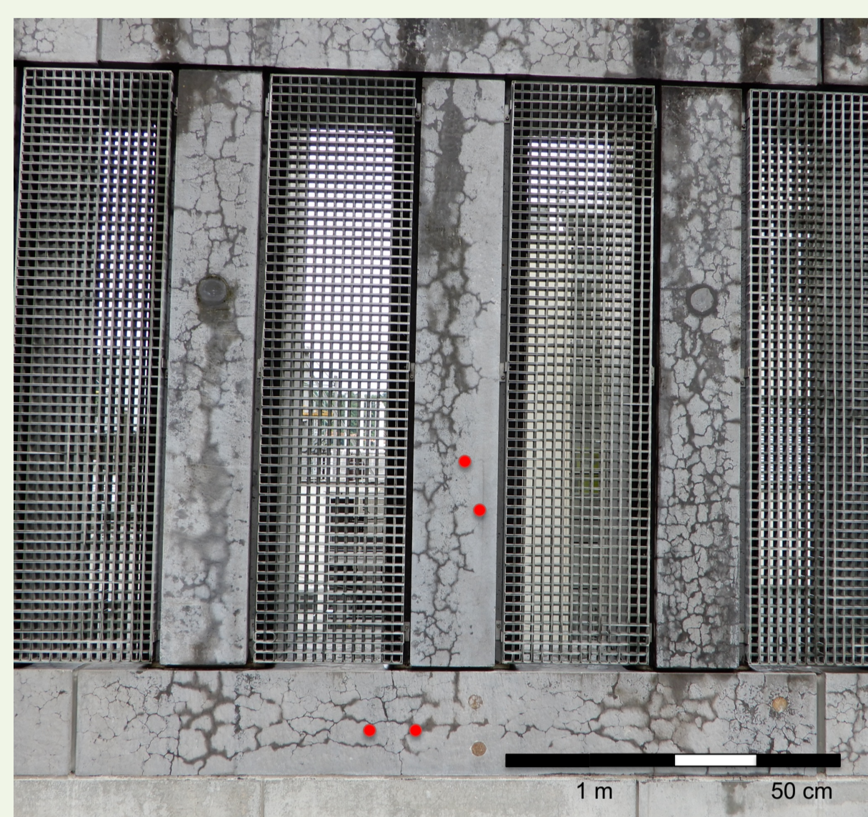
Figure 1: Concrete precast elements of a damaged building wall with the collected drill core samples in red.
